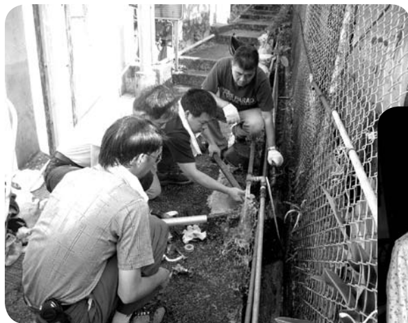
義工正為李伯伯接駁水喉 Volunteers Installing Water Pipes for the Lee's
